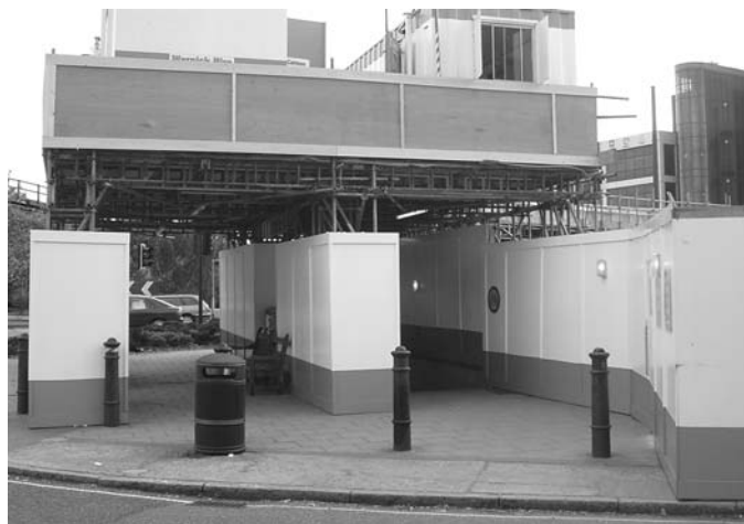
Fig. 2.12 Hoarding encroaching onto footpath with site offices above
